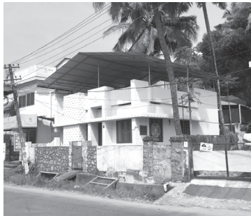
4. Mrs. Elizabeth Jose, Peroorkada, Member. Bills to be settled Renovation work, nearing completion
